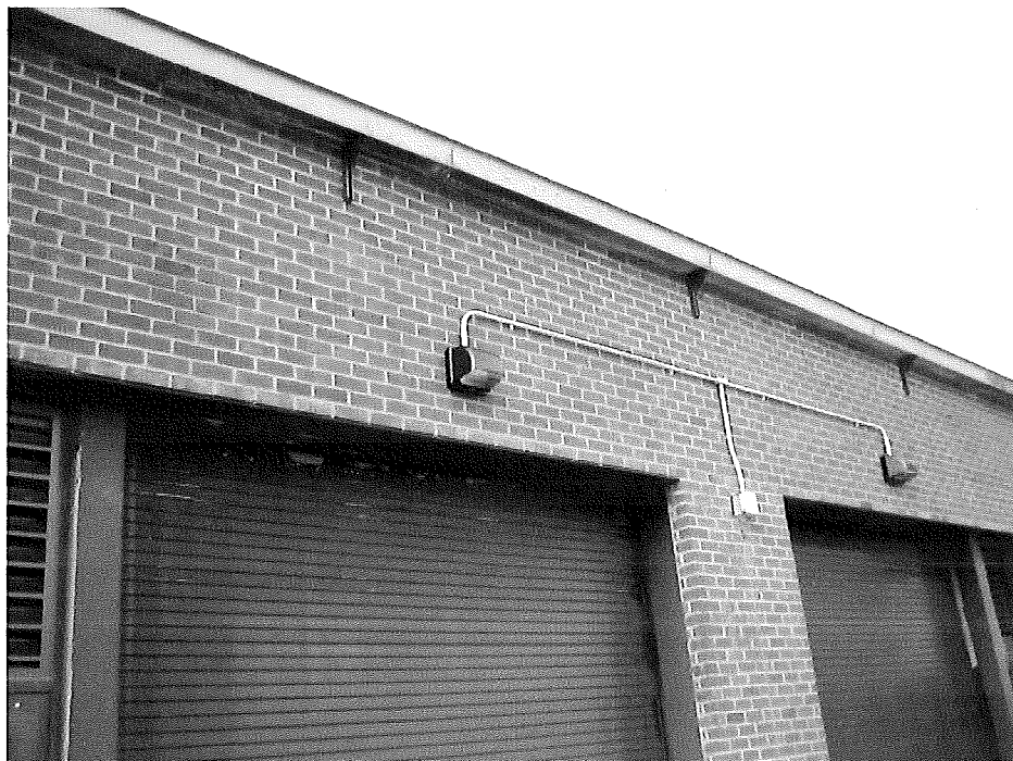
3 gutter supports installed in November to restore proper draining and lessen ice accumulations.
