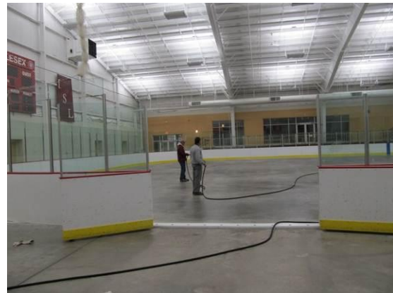
Under the new lighting, Middlesex School staff builds the rink's ice surface
