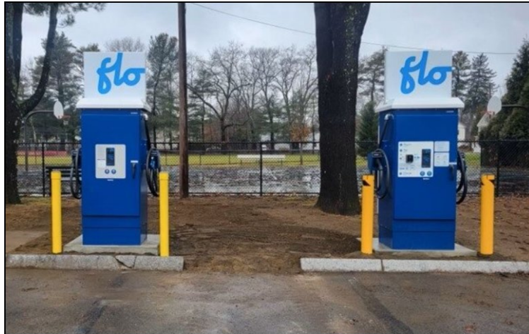
Figure 2: Flo chargers installed at the Rideout Park
